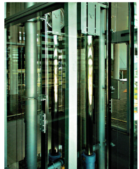
Panorama lifts with parallel-positioned single-stage jack.
